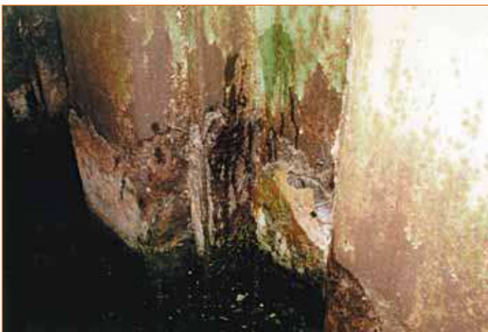
FIGURE 10 - Corrosion de palplanches.
